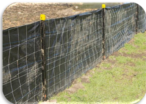
Silt fence staked and trenched into ground. For more information about use and installation see the "Silt Fence Barriers" brochure or contact the Stormwater Department.
